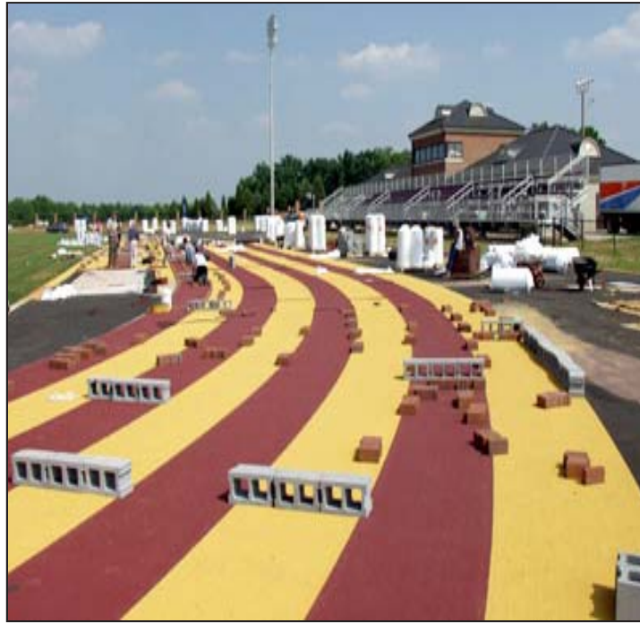
Work continues on Winthrop's new outdoor track, currently being built by Farley Construction Company near the university's golf course. The $2.8 million project will give Winthrop an NCAA Division I competition track with a top-quality Mondo rubberized surface. The track will encircle a full-sized practice field for soccer, as well as areas for field events, such as discus and pole vault. Here, concrete blocks stabilize the surface, helping the sections bond to each other.
